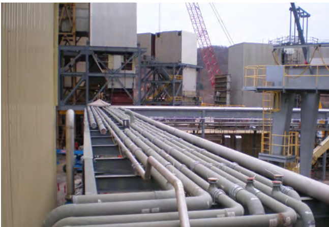
HPPE A-150 in service as CCR piping at a US power utility.
