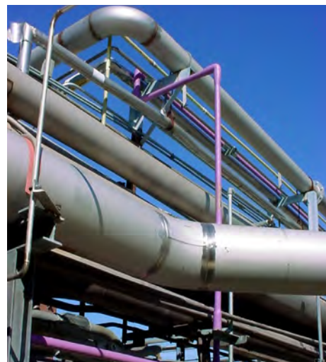
Installed system for hypochlorite in service since 2000.
