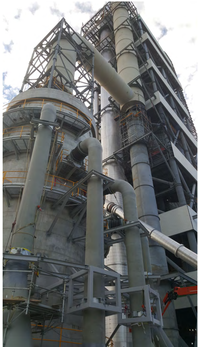
HPPE A-150 in service in a flue gas desulfurization process.
