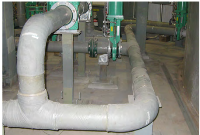
HPPE A-150 in service as FGD process pipe at a US power utility.
