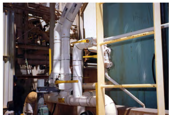
Minimally flanged installation for sulphuric acid in service since 1996.
