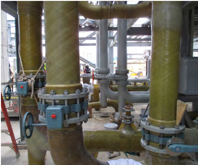
HPPE P-150 in service in a cooling water unit.
