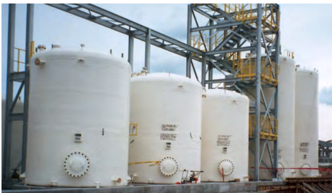
PP-lined phosphoric acid storage tanks
